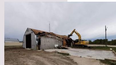
Demolition of the old grader shop and public works building was completed in September.
